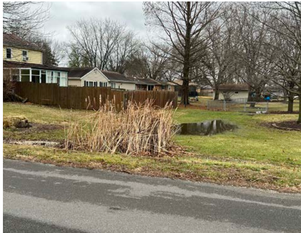
Drainage issues South of Dunbar St.
